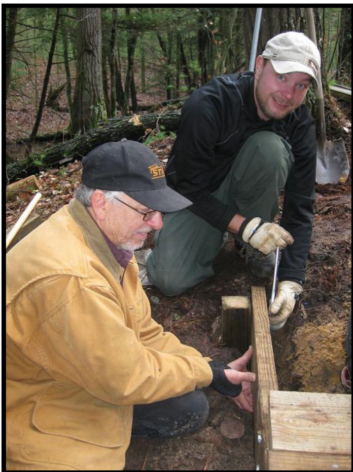
WMI Volunteers Larry Meyer (left) and Gareth Hickson work on the decking for the south approach to the Cole Creek Bridge.
