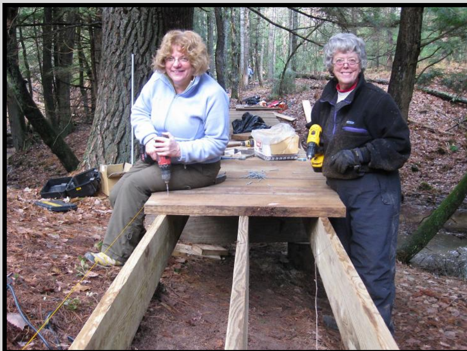
WMI Volunteers Joni Hernandez (left) and Pam Stonehouse work on the decking for the south approach to the Cole Creek Bridge.
