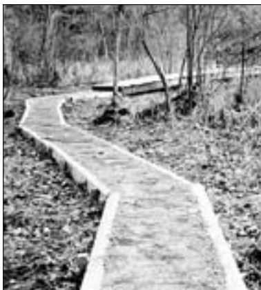
A section of turnpike built in the wet areas leading to the bridge at Bigelow Creek. PHOTO BY AARON PHIPPS
